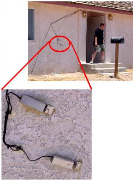
Figure 1 Test House Showing Closeness of Construction and Sensor Across Crack 2
